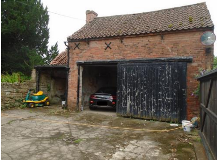
2016 Photograph of the collapsed building
